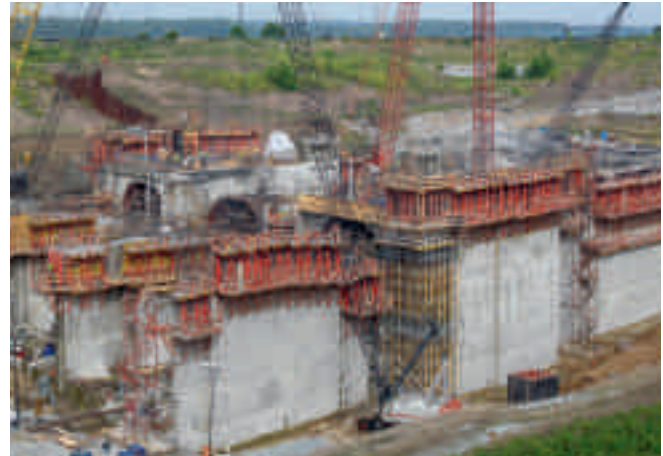
The massive power plant walls were single-sidedly formed and concreted using the SCS Climbing System.
