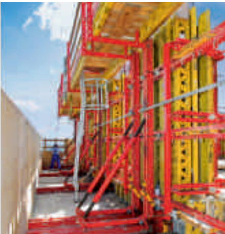
This column formwork in the facade area climbs crane-independently upwards with the RCS Self-Climbing Technology. At the same time, the enclosure provides protection against wind and weather.
