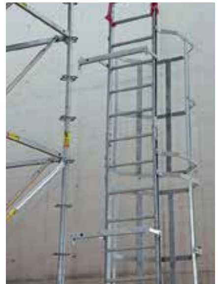
Lifted into position by crane, the wedges are then fixed using a hammer.
